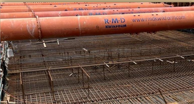
Substructure construction at MBR Treatment Facilities 薄膜生物反應處理大樓地下結構工程
