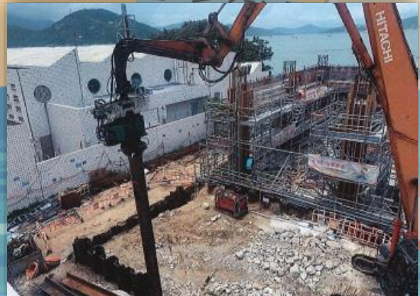
Sheet Piling Work at Sludge Digester Building 污泥消化大樓板樁工程
